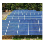
26001 On - Grid Solar Power Plant
