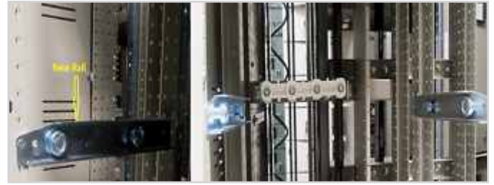
Power & Control Connections
